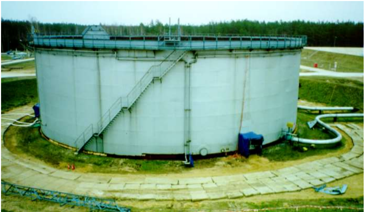
Fig. 2. General view of the tank
